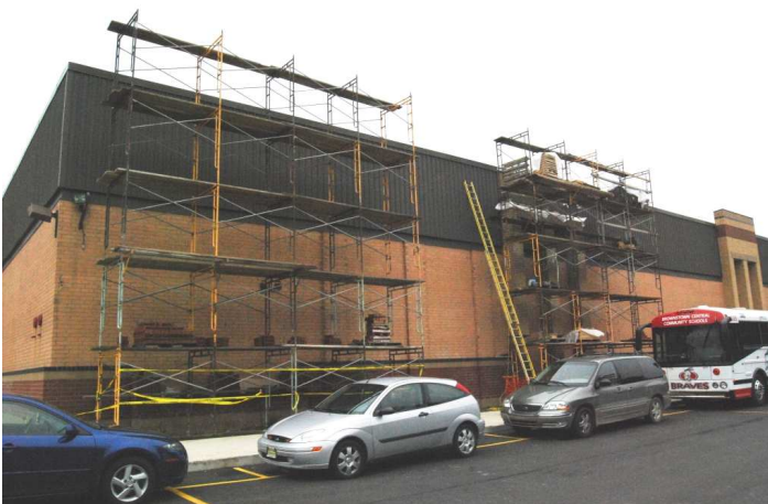
While many areas of construction for Phase 2, some touch up does continue without interfering with the school’s day-to-day operations.
